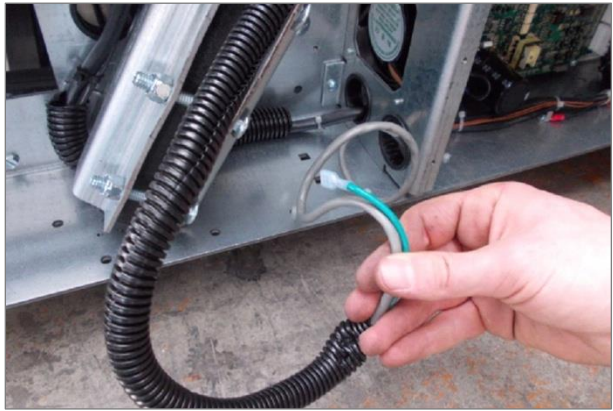
Fig. 43 Mercury/Path assembly, connection 1
